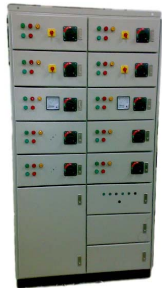
Main Control Panel
